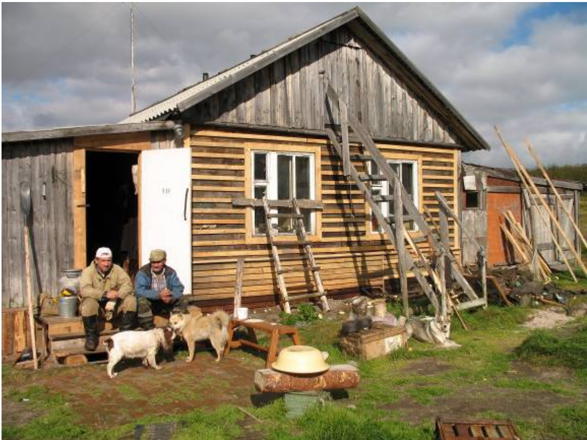
Picture 2. The summer of 2007 was marked by long needed repairs to tundra base camps. Renovation and re-insulation of walls at the Kolmiavr base camp of Brigade 8.
